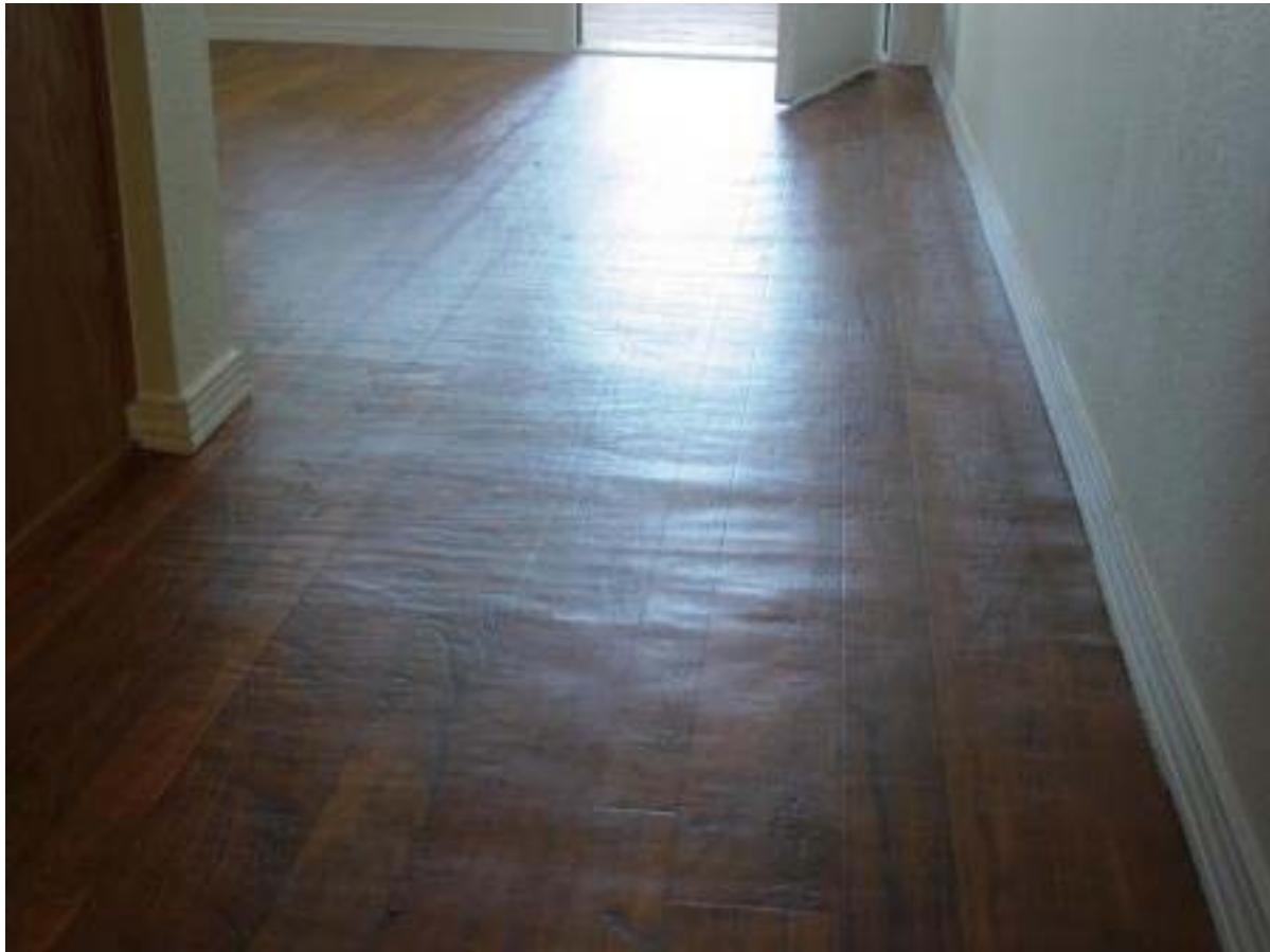
Figure 2 – Buckled floor at Parris Island home.
