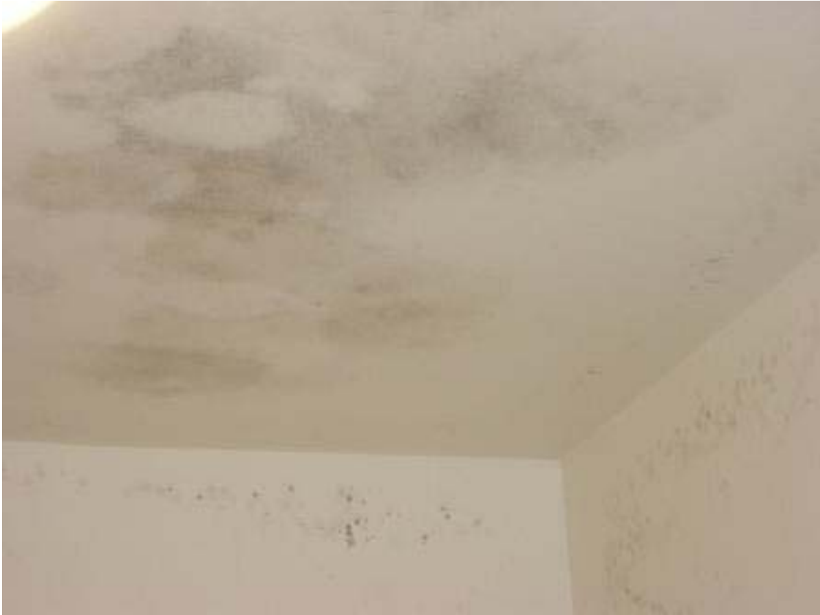
Figure 3 – Visible mold on ceiling and top of walls in bath.
