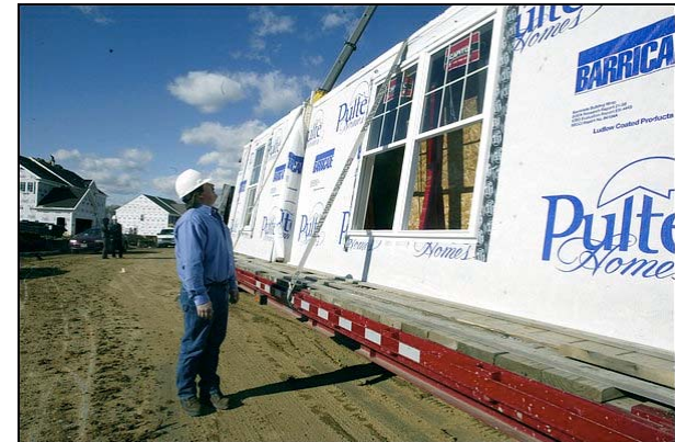
Prefabricated wall panel being set on a site Source: Washington Post, Photo by James A. Parcell
