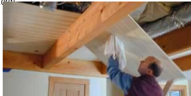
Accessible Ceiling Panels
