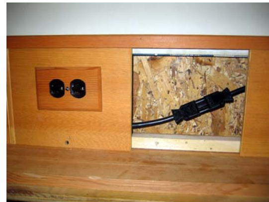
Baseboard molding with recessed, accessible chase for electrical lines
