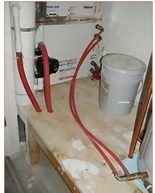
The GHP manifold with circulatory pumps connect to the home's HVAC unit.
