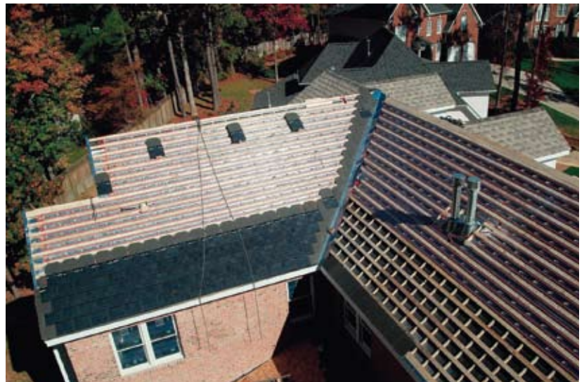
The solar panels on the Mainstream GreenHome take on the look of traditional shingles, enabling the energy-producing roof to blend in with the others on the block.
