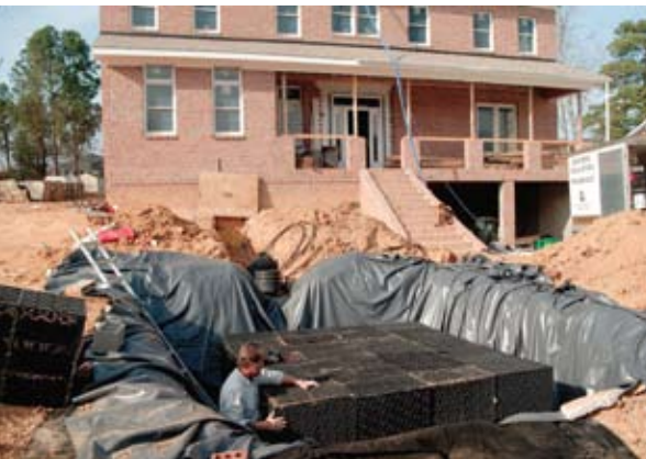
Rainwater is harvested from the roof and stored in an underground cistern to be reused for toilets, laundry and irrigation.
