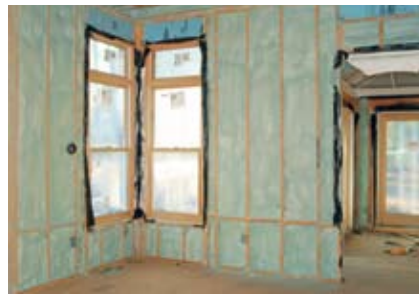
The spray foam insulation in the home expands 30 times its original size upon application, helping create a tight seal for an energy-efficient building envelope.
